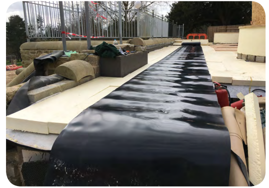
Newton 409 RootBarrier was installed as a final line of protection beneath the above-ground landscaping
