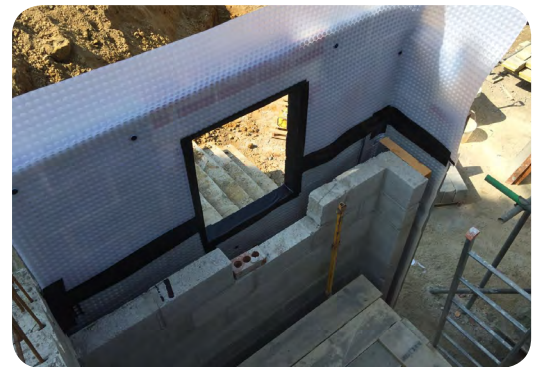
A blockwork lining wall was constructed internally inside the full System 500 cavity drainage membrane
