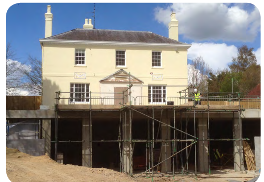
The extensive basement area was a large-scale extension to an existing property
