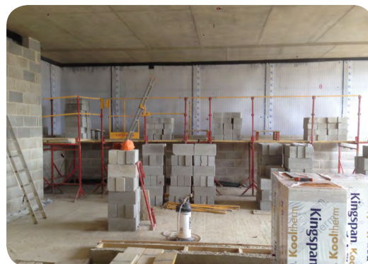
Newton System 500 was installed to the internal wall and floor areas to provide full internal protection
